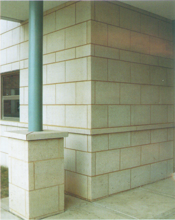
Rochester Century High School, Rochester, Minnesota Architect: Hammel Green and Abrahamson, Inc. Block Color: Parchment
